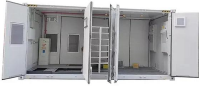
1075KW HH ESS
