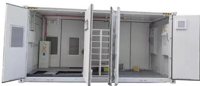
1075KW HH ESS
