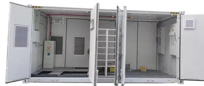
1075KW HH ESS
