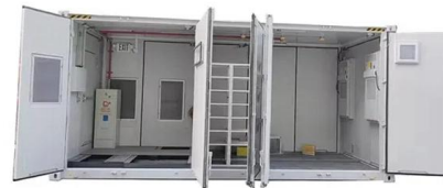
1075KW HH ESS
