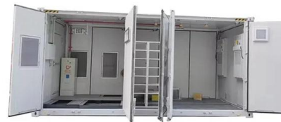
1075KW HH ESS
