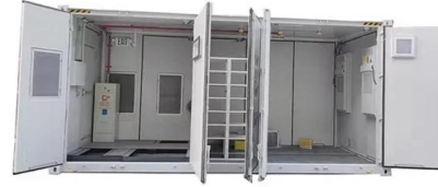
1075KW HH ESS
